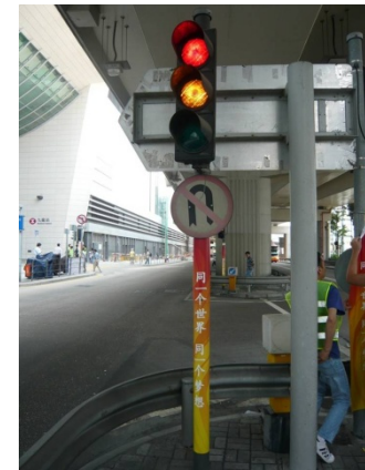
Traffic signal poles
